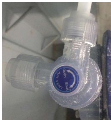
Figure 12: Bouchon pompes doseuses
